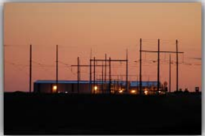
Tatanka 230 kV substation
